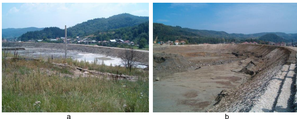
Fig. 6 The basin for taking over the brine waves: a - general view; b - structural degradation of the dam under the action of sodium chloride (Luca and Tigaret 2008).
